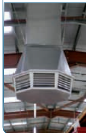
Above, centre and below: installing evaporative cooling is low cost and very effective
